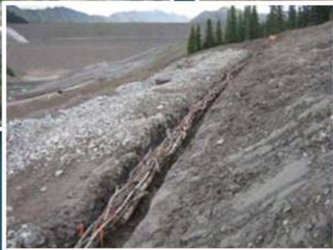
Borrow 10: before (left) and after (right contouring); Live pole drain at Borrow 10 (center)
